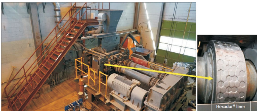
Figure 1. Photos of the Köppern pilot-scale high-pressure grinding roll (HPGR) unit installed at The University of British Columbia: left) the pilot-scale HPGR unit; right) close-up of the HPGR roll's liners.
